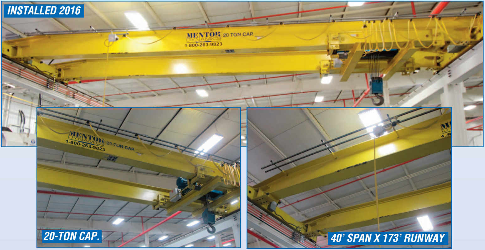
MENTOR DYNAMICS FREE STANDING BRIDGE CRANE SYSTEM (LOCATED IN ST. THOMAS, ON)
